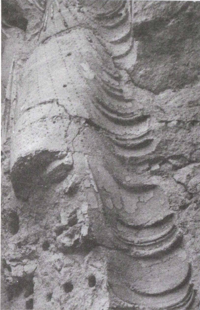
15. Right thigh of the Big Buddha showing cracks.
