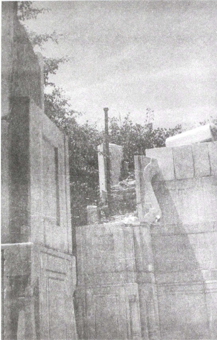
44. A portion of Shahjahan's mosque showing repairs near the tomb of Babur.
