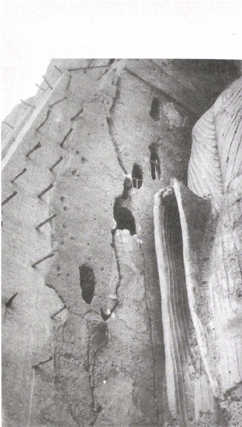
18. Cracks on the western wall of the niche of the Small Buddha.
